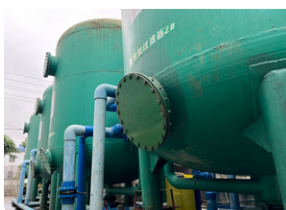
Final filtration tanks
